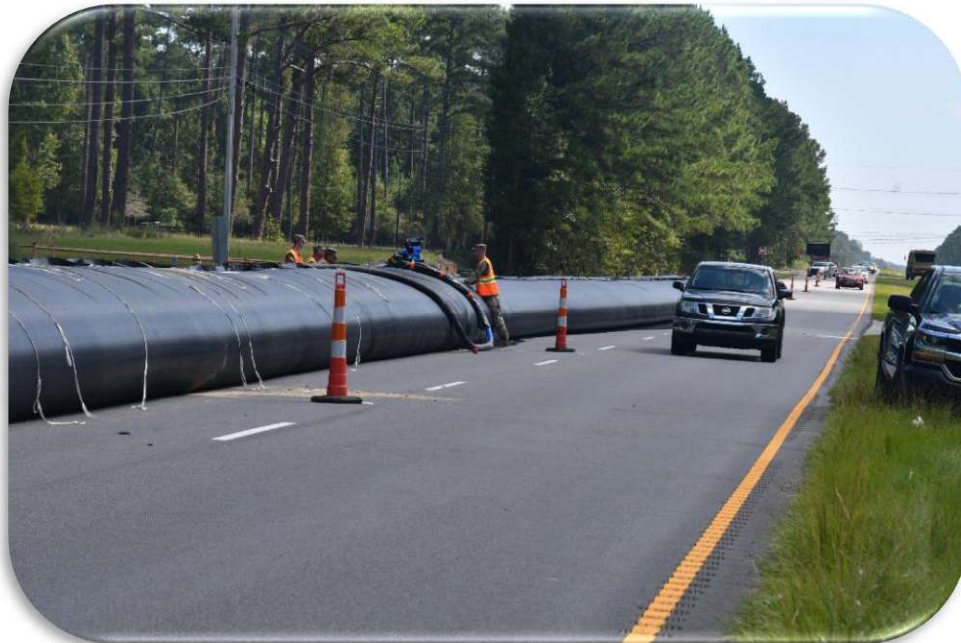
Figure 3.5 – Example of Temporary Flood Barriers
