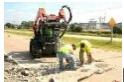
Example of buckling on Highway 16 in Portage, Wis.; Photo credit: PORTAGE DAILY REGISTER ARCHIVES
