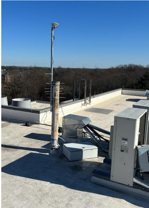
Figure 3. GNSS antenna installed on the roof of McEniry Hall on UNC Charlotte's main campus. (Image courtesy of Beep)
