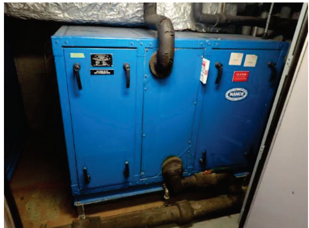
Second part of central HVAC system onboard older vessel
