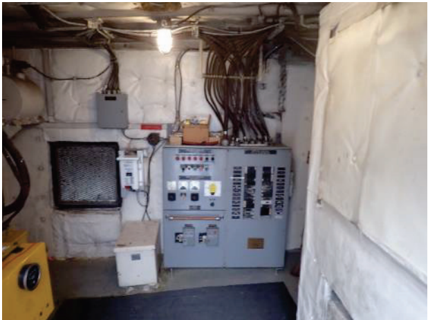
Typical electric sub panel and cables.
