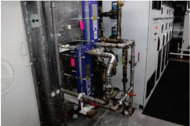
New vessel piping and coolers
