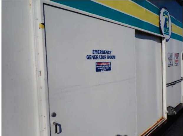
Example of emergency generator access door
