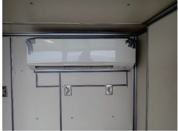
Mini split showing susceptibility to damage
