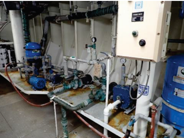
Potable water piping and pumps
