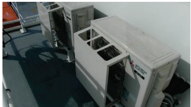
Newer mini-split systems installed
