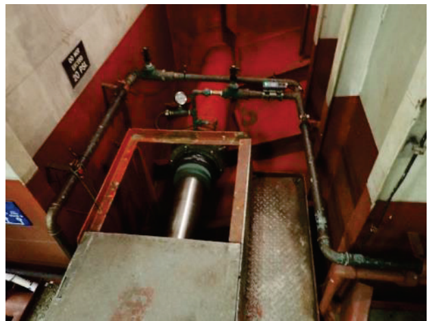
Shaft in engine room and shaft seal
