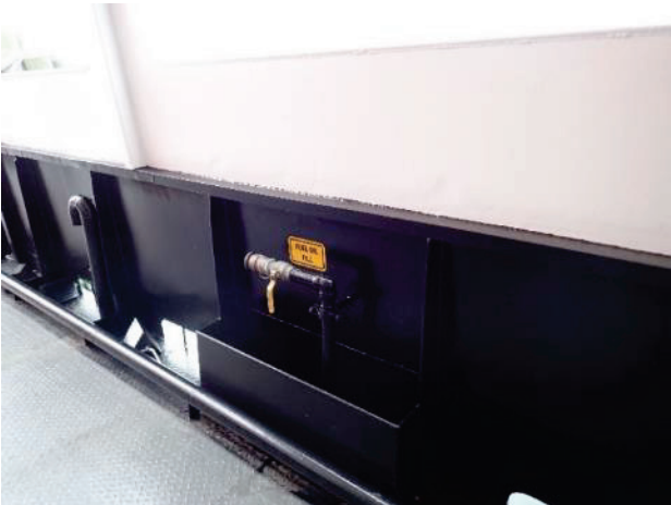
Typical piping on deck area
