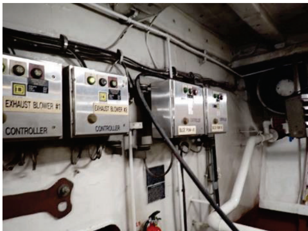
Condition of some controller panels.
