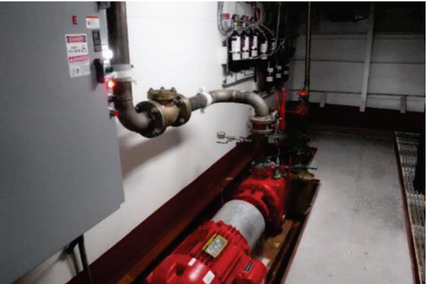
New vessel piping and fire pump
