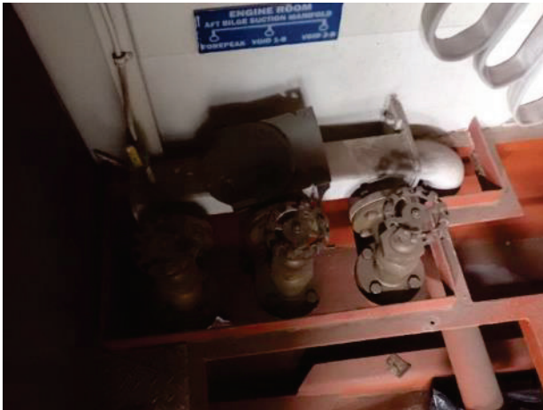
Valves for bilge system
