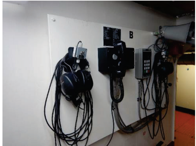
Communications arrangement on mid age vessel
