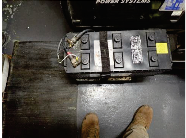
Starting battery for emergency generator.
