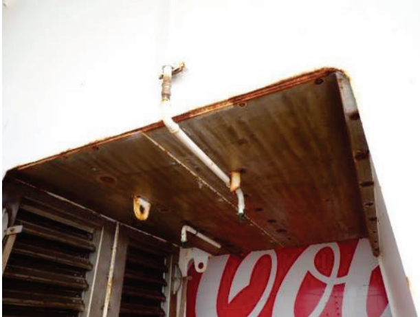
Typical corrosion under deck of Sound Class vessel
