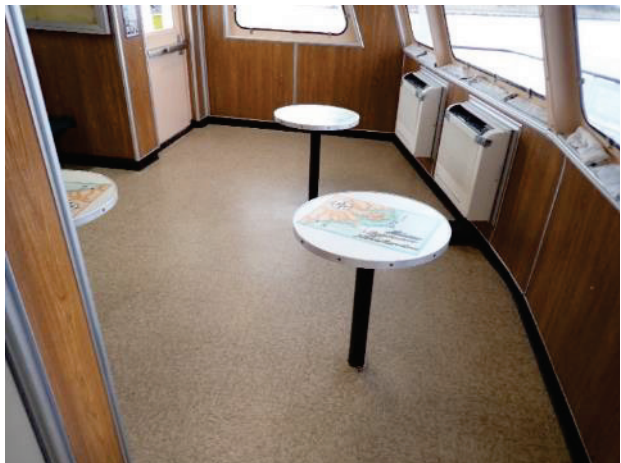
Mid aged Sound class vessel with leaking window
