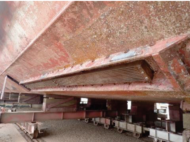
Depleted zinc anodes on keel cooler of hull.
