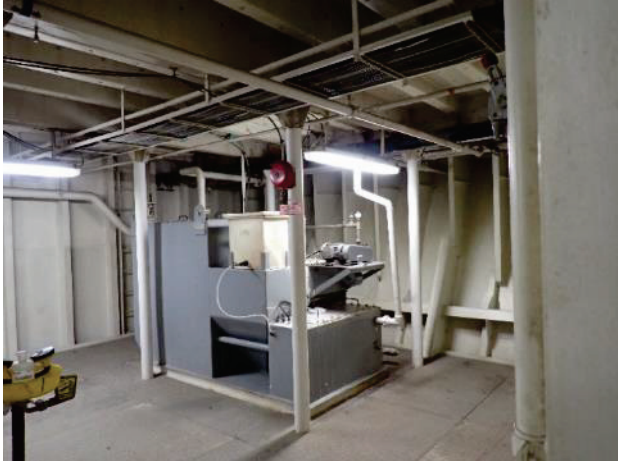
Sewage treatment system on older vessel
