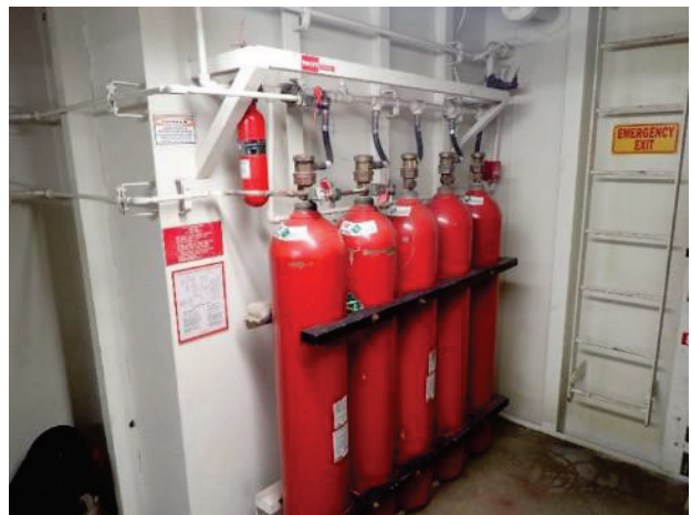
Older CO2 fixed fire fighting arrangement
