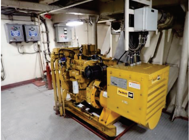
Typical Caterpillar auxiliary generator
