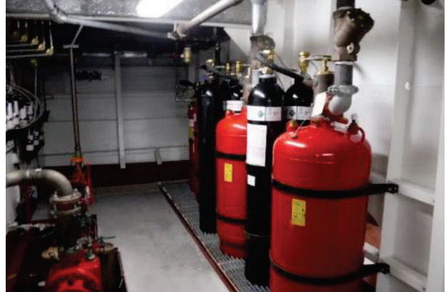
Newer fixed firefighting and fire pump
