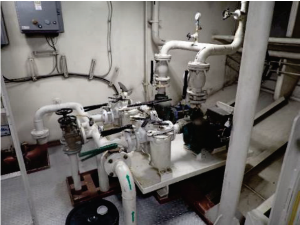
Sea water pumps and piping system
