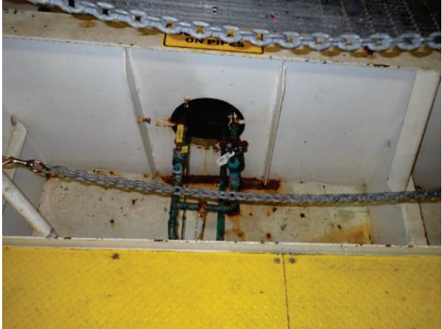
Piping in bilge area
