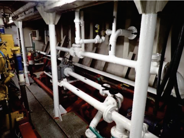
Piping in engine room showing maintenance done
