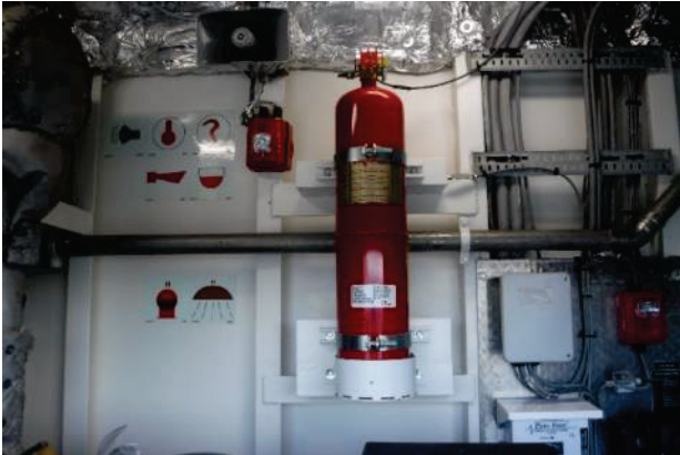
New vessel fixed firefighting set up
