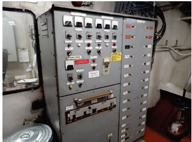
Switchboard of medium age
