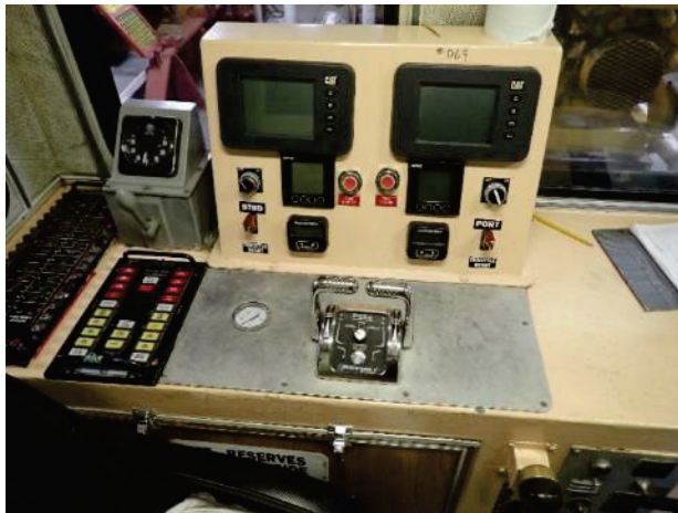
Older style engine control with Caterpillar engine controls
