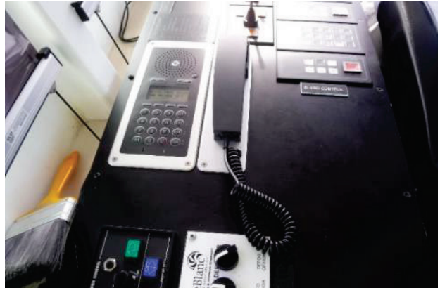
New vessel electronic telephone
