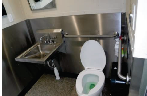
New vessel passenger accessible head stainless on bulkhead and terrazzo type deck
