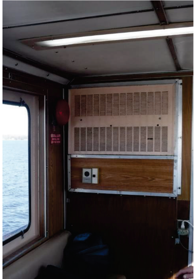
Typical central HVAC system register
