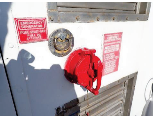
Typical emergency shutoff for E-Gen Fuel oil
