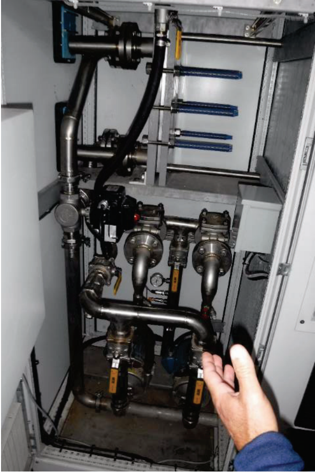
New vessel piping
