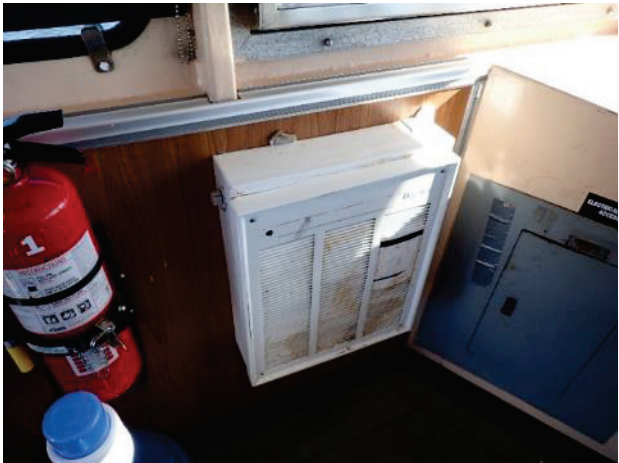
Electric heater on older vessel
