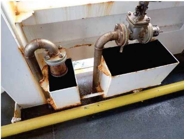
Piping, vents and containment on deck
