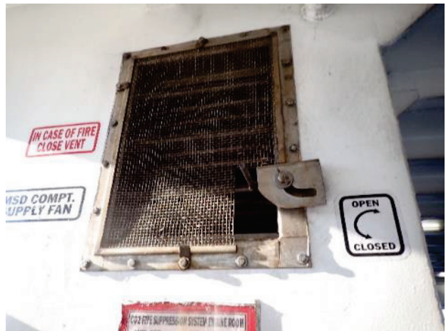
Typical condition of emergency vent and closing apparatus
