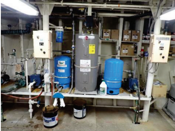
Another potable water system with piping pumps, pressure tanks and heater
