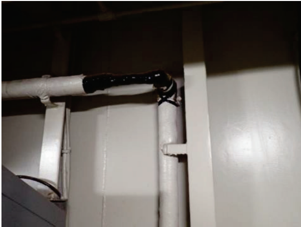
Example of piping insulation repaired with vinyl tape
