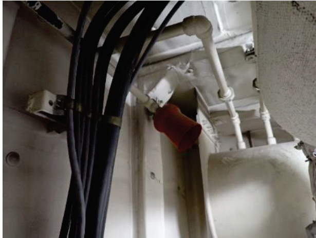
Typical cables mounted on bulkheads
