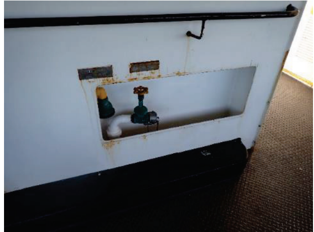
Moderate corrosion in way of superstructure opening
