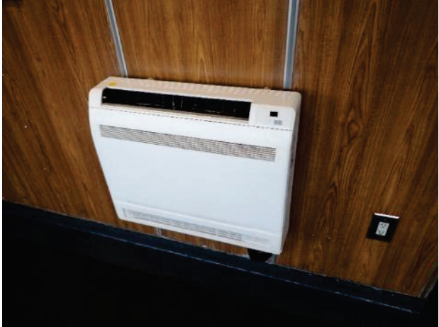
Another view of mini split in accommodation
