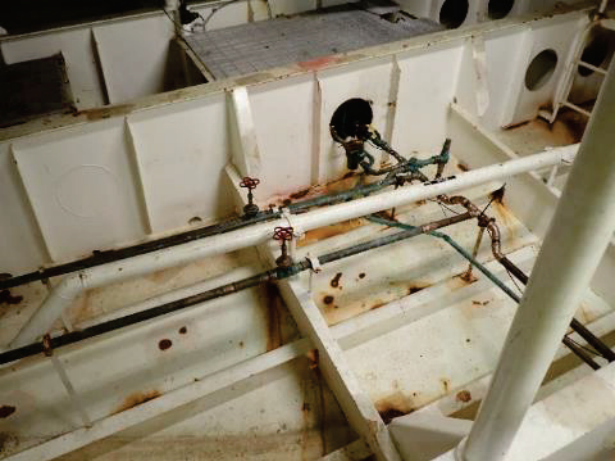
Piping in bilge area
