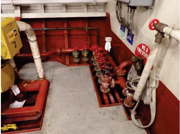
Different valve and piping arrangement for engine room bilge area
