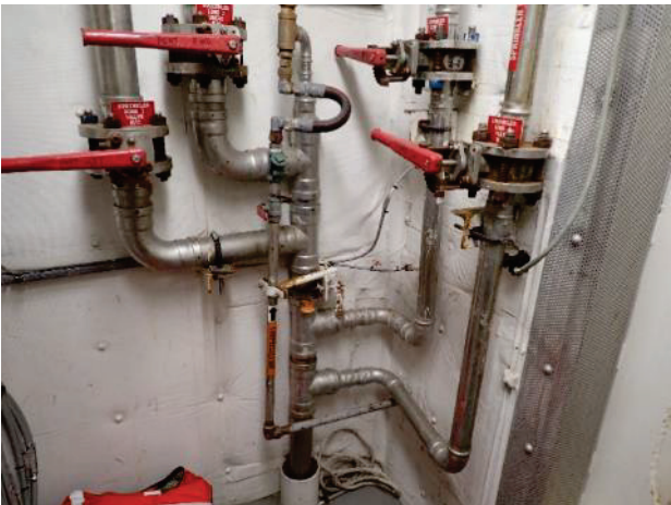
Firefighting piping installed
