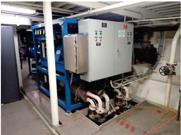
Central HVAC unit onboard older vessel
