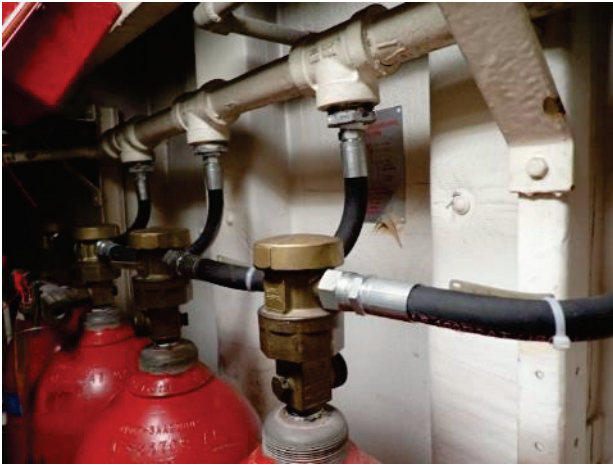
Fixed fire-fighting CO2 hoses in very good condition
