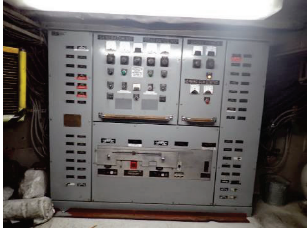
Very old switchboard from Gov Hunt
