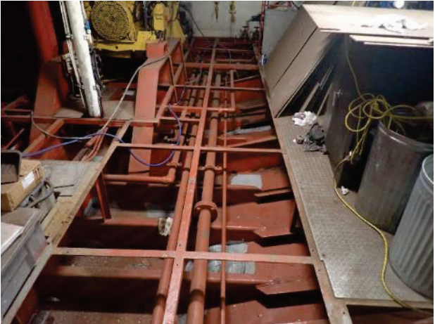
Bilge condition typical
