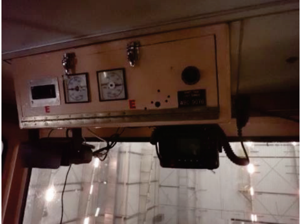
Older VHF radio install
