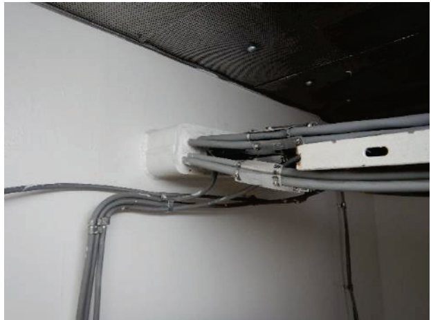
Newer vessel cable and bulkhead penetration
