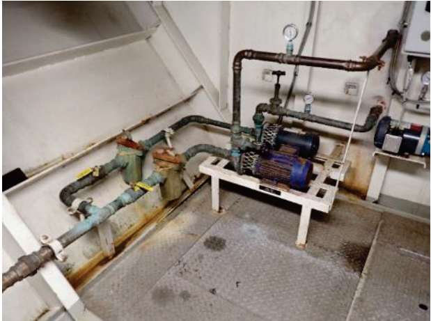
Water pumps and piping systems as typical
