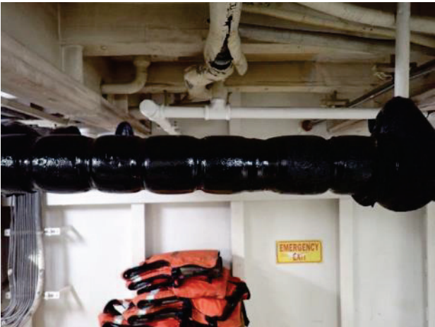
Piping with valves and insulation
