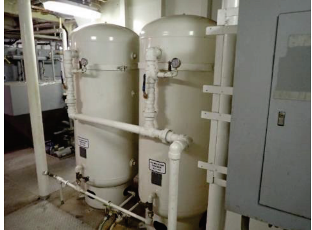
Typical air receivers installation
