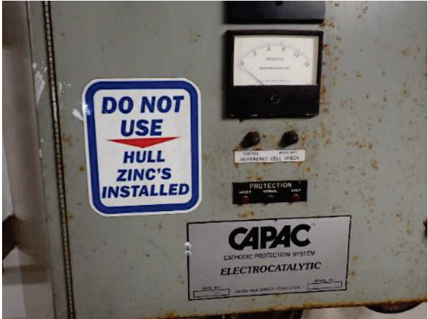
CAPAC systems have all been decommissioned in favor of hull zinc anodes
