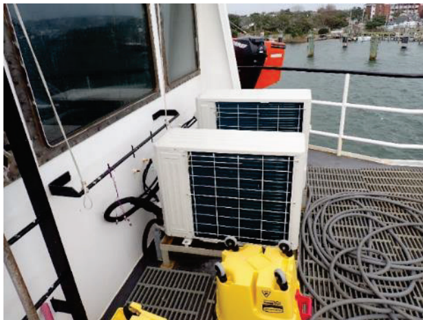
Mini split HVAC systems for upgraded pilot house
