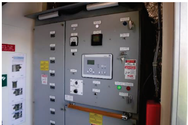
Newer vessel switchboard example
