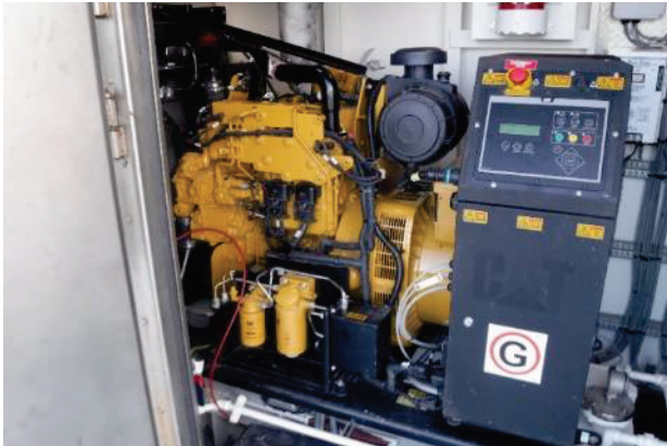
Newer vessel emergency generator
