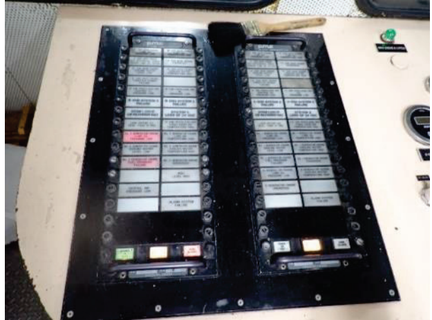
Typical alarm panels on bridge
