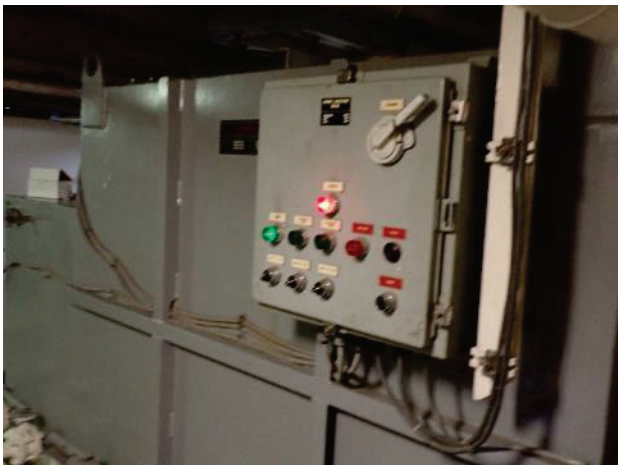
Red Fox sewage treatment system
