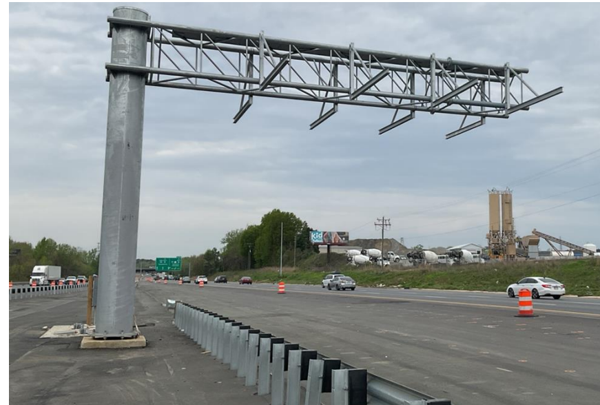
Express Lane Gantry at Site 1
