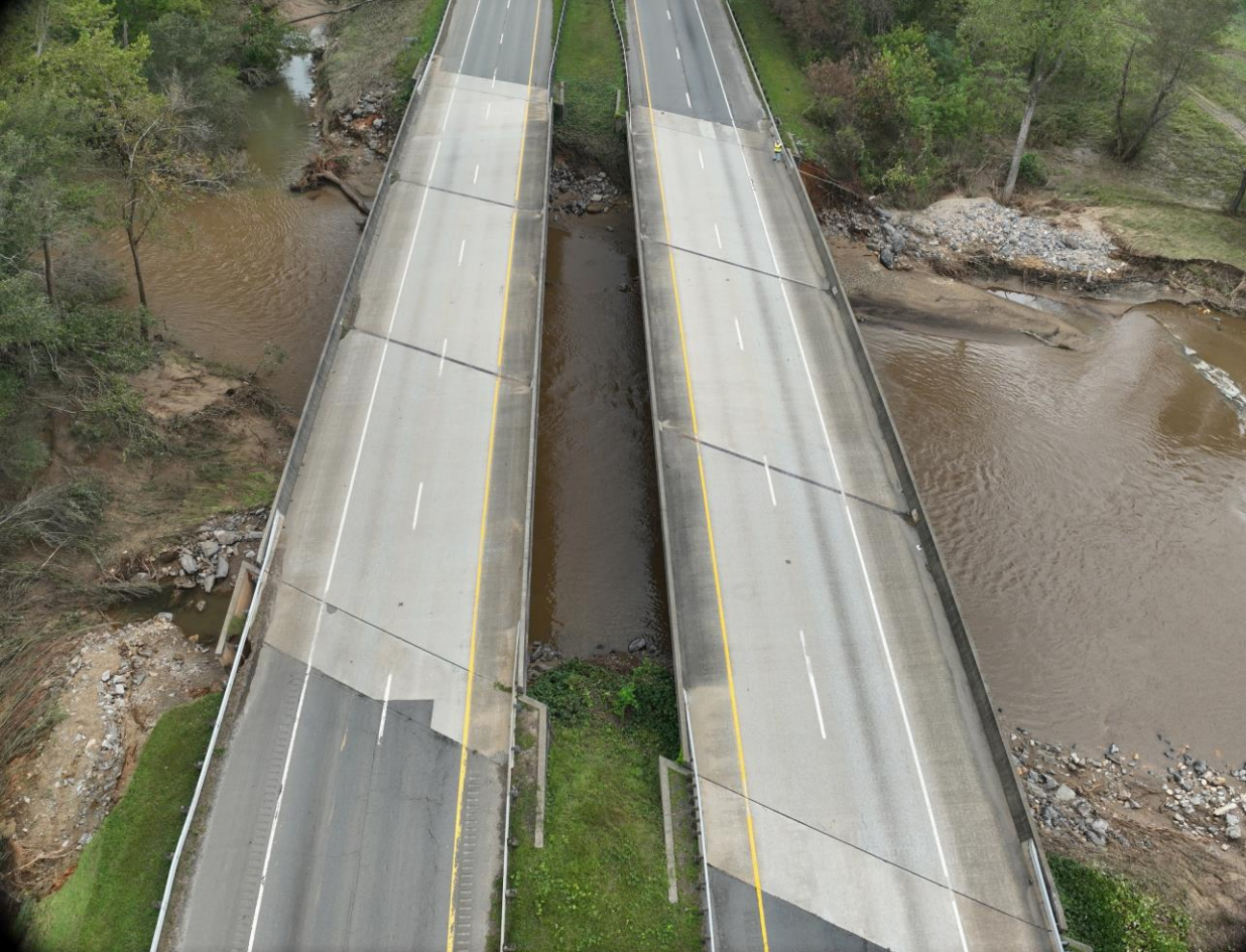
UAS team on TSMO Unit mission discovers compromised bridge with massive scouring, still fully open to traffic
