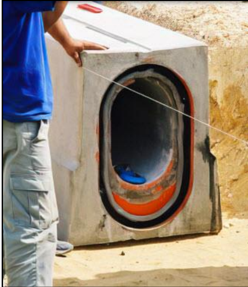
Installation of CS-440 on concrete pipe joints during installation of a stormwater drainage system at Ben Gurion International Airport in Tel Aviv, Israel – image from ConSeal™ website
