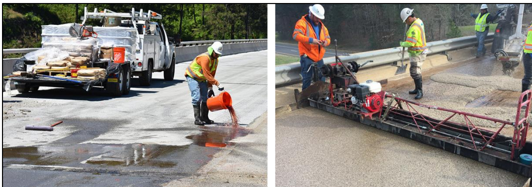
Worker pouring and rolling primer resin on the bridge deck (left), Workers pouring and leveling PCC 1121 on a bridge deck after the primer is applied (right) – images from Kwik Bond Polymers website
