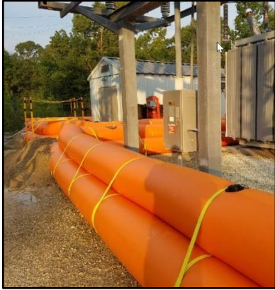
Tiger Dam™ protecting an electrical substation prior to flooding – image from U.S. Flood Control Website
