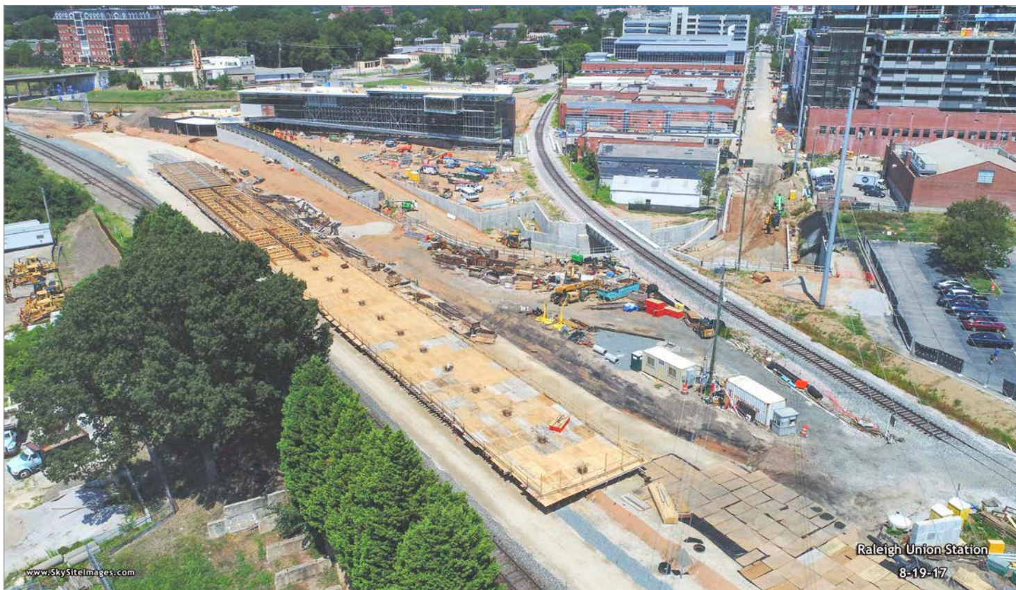
View of south elevation with passenger concourse (center of photo), and footings for high-level center island platform (left center of photo)
