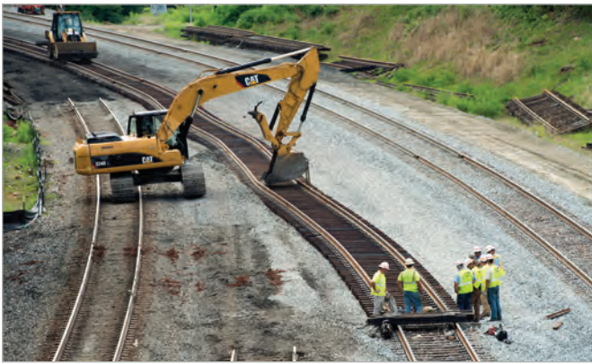
Previously passenger trains had to slow down to 45mph in Duke Curve. This curve realignment project allows passenger trains to travel up to 65 mph.
