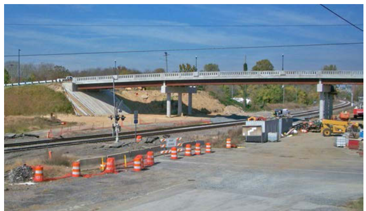
Roadway improvements included in the B-3421 bridge replacement project allowed the Corban Ave crossing to be closed.
