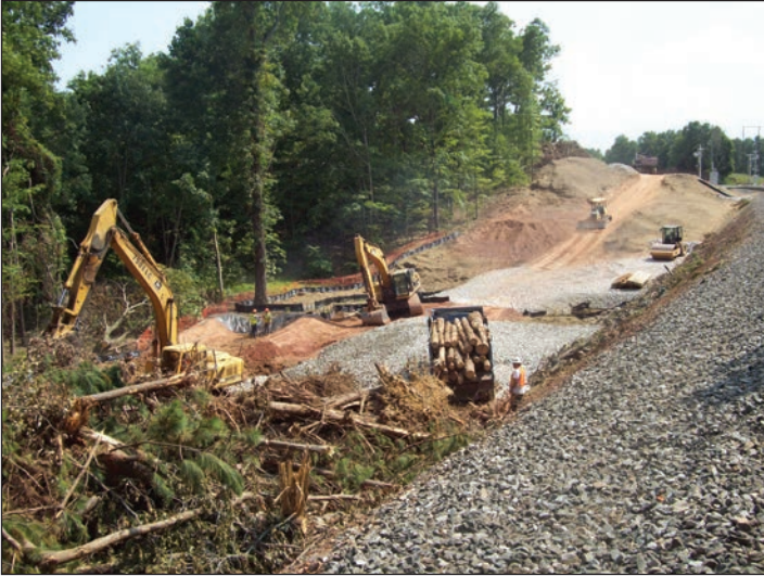
P-5201 Morrisville Parkway grade crossing erosion control
